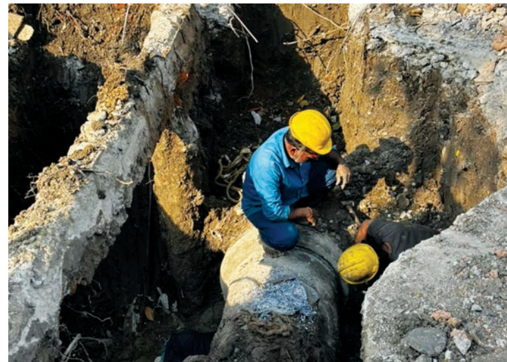
Officials revealed that a detected leakage in the main water supply pipeline, combined with the improperly constructed toilet, created conditions for sewage to contaminate the drinking water supply.
