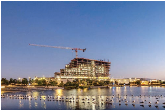
Kali Hotel at Hollywood Park: the ceremonial raising of the final structural steel beam.
